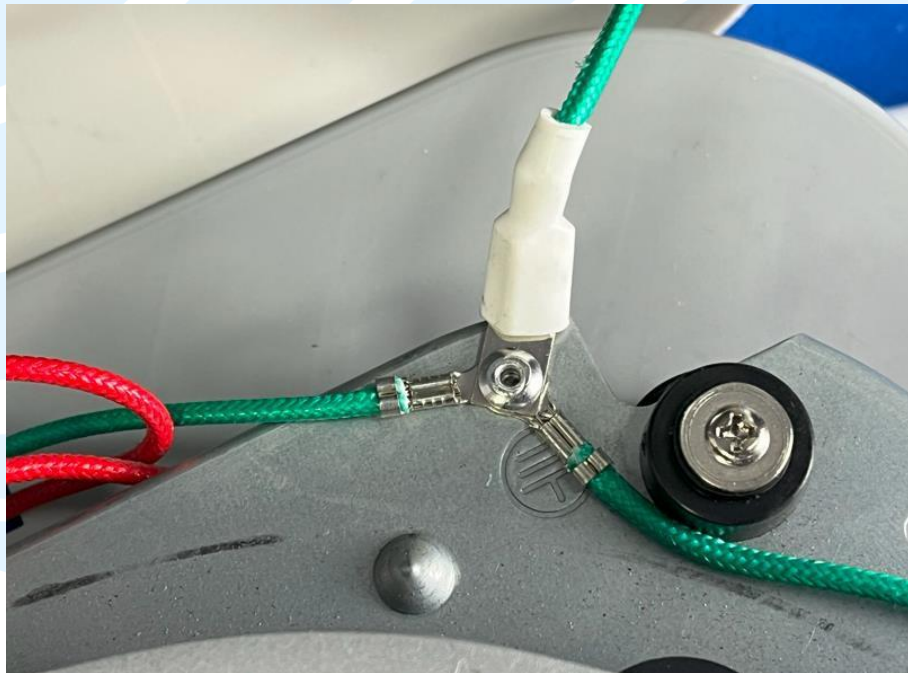
Description: Earthing terminal - CY01
